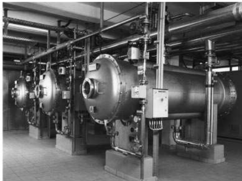
Figure 14 Ozone generators for water treatment [10].
