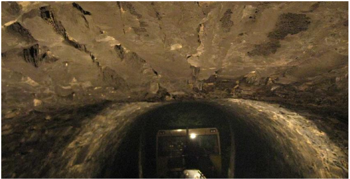
Obr. 2-4: Deformace klenby v pasu T10 [13]
