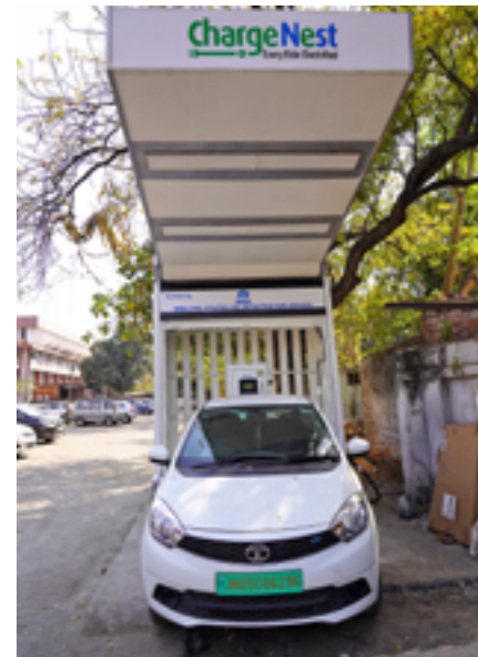
Nest-In's ChargeNest Electric Vehicle charging station in Jamshedpur
