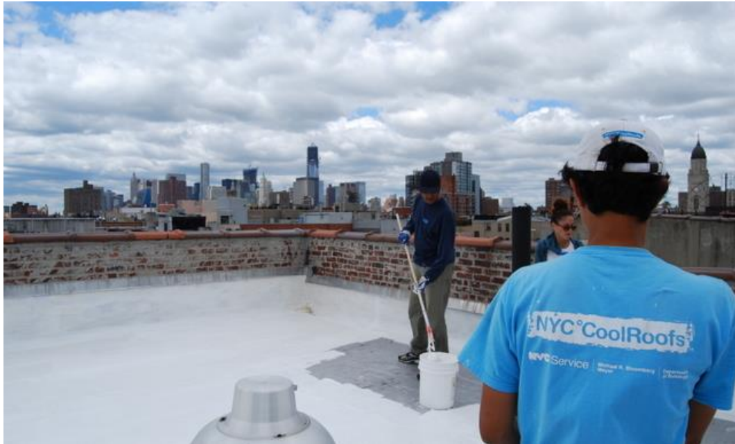
Figure 3: Project staffs are painting dark roof to white in NYC (Ben Huff 2012).
