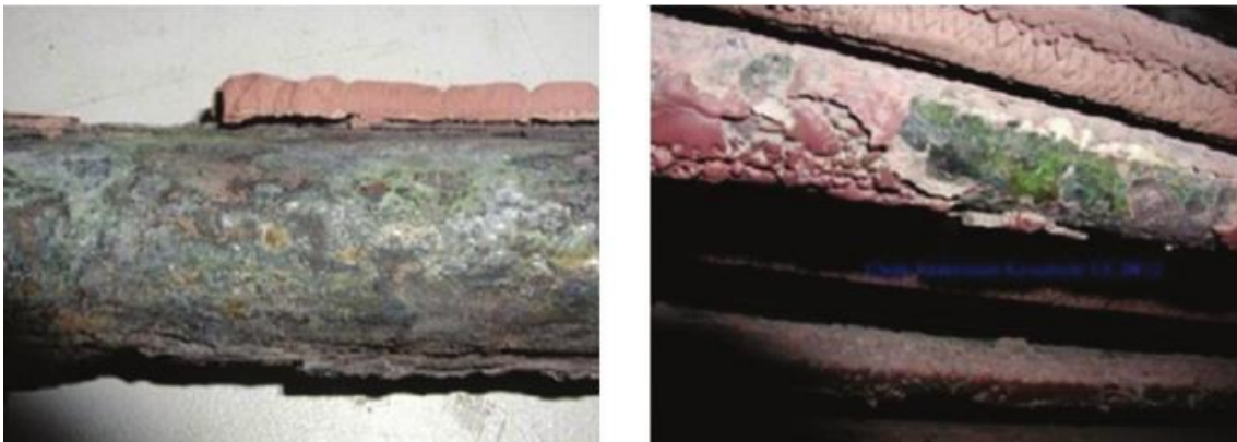
Figure 9. Corrosion from using a high chlorine biomass.
