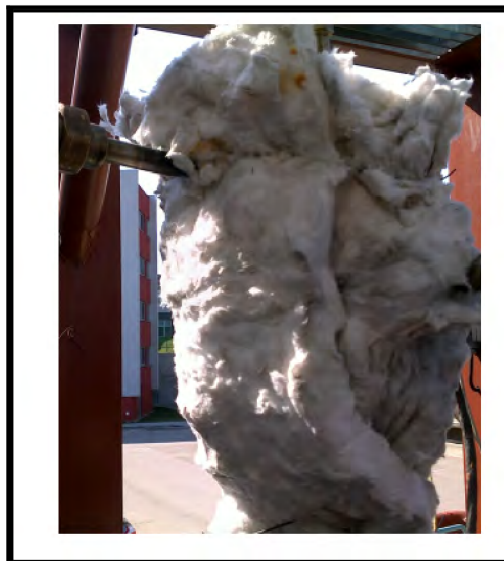
Figure 8.8 Filter after installment
