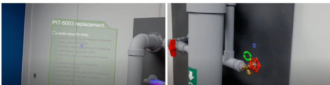
Figure 3.1: Left: A list of tasks is rendered directly in the user's view and can be moved to a different position. Right: Rendered AR elements have specific meaning 2 .
