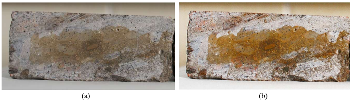
Figure 37: Sprayed specimen with \text{AgNO}_3 solution after splitting test used for in the measurement of the chloride penetration dept – (a) original photo (b) adjusted photo with more clear boundaries of the chloride affected surface.
