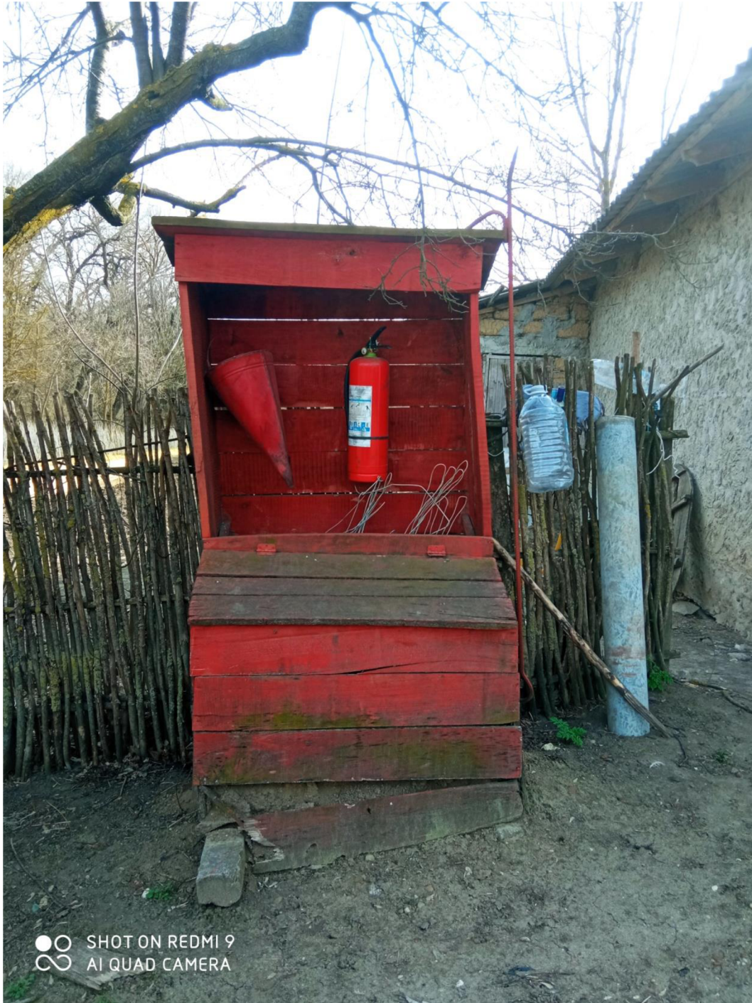
Photo 14. Emergency fire box from the Forest range Nr.2
