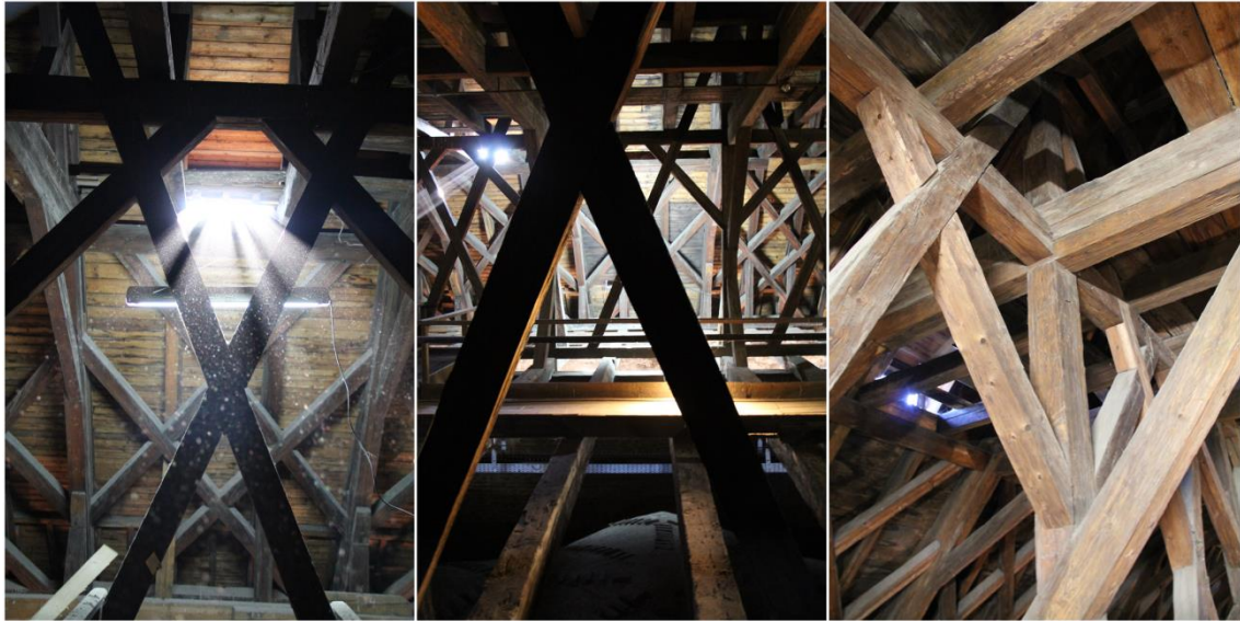
Figure 2: Truss structure of St. James's Church; left: details view into structure with St. Andrew's cross-like members, right: details of beam connections in the structure.
