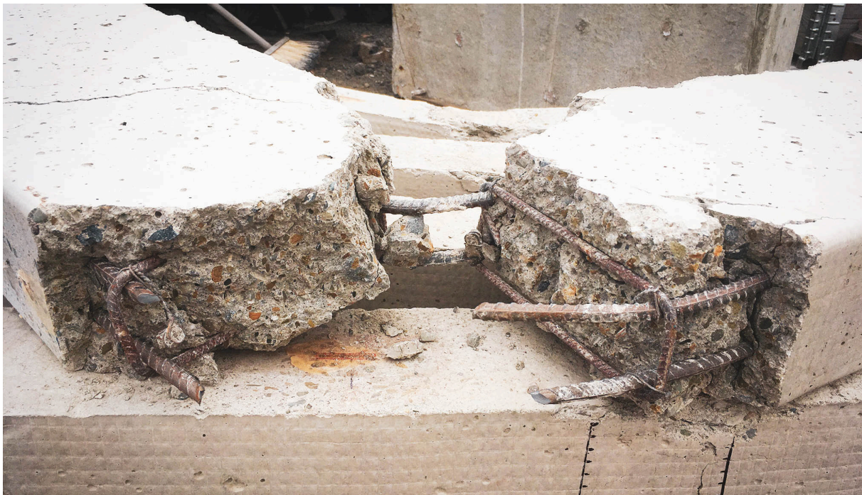
Fig. 8.7. Damaged specimen 7IX-4 after the second impact (post-critical damage).
