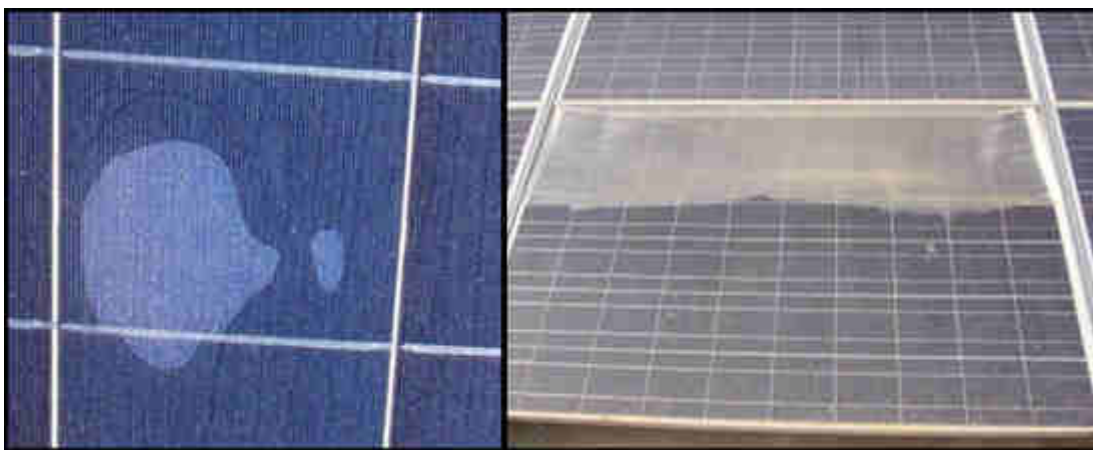
Obr. 2.2-3 Delaminace FV panelu [11]
