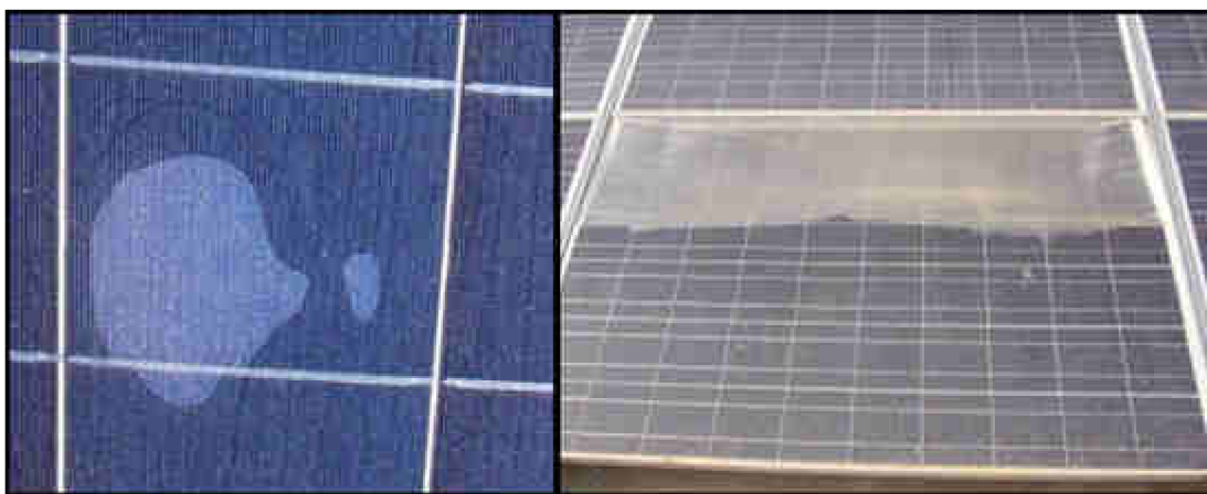
Obr. 2.2-3 Delaminace FV panelu [11]
