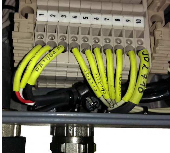
Fig. 3.1: AWS receiver's junction box.
