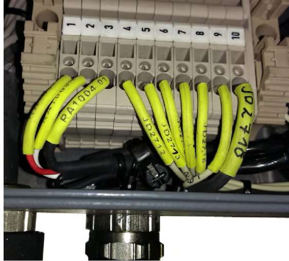
Fig. 3.1: AWS receiver's junction box.
