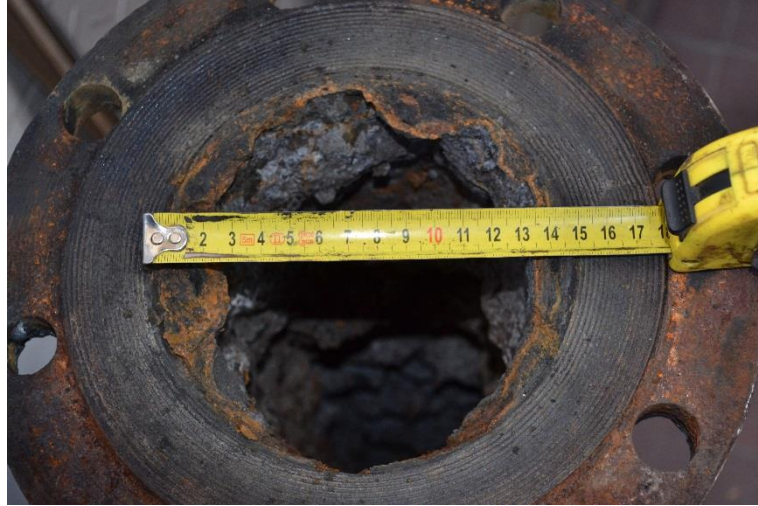
Picture 3.27. – Sedimentation incrust at inner pipeline perimeter
