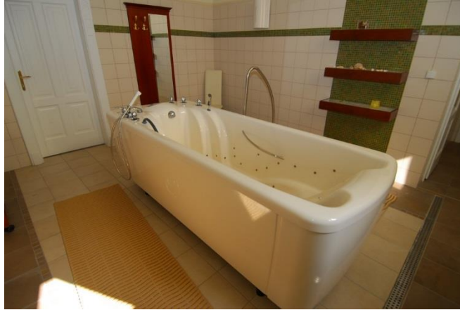
Picture 3.13. – Bathtub for water treatment
