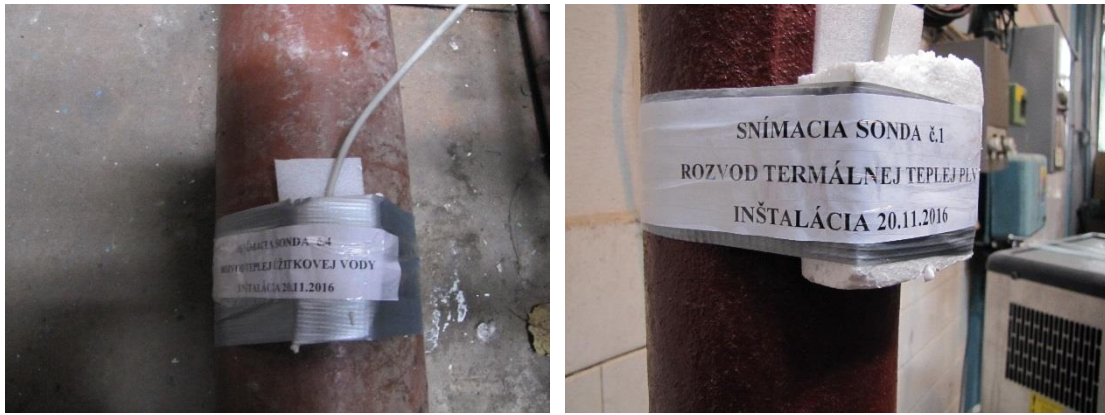
Picture 3.26. – Left: Temperature sensor at hot service water (yellow pipeline), right: Temperature sensor at hot natural healing water (red pipeline)
