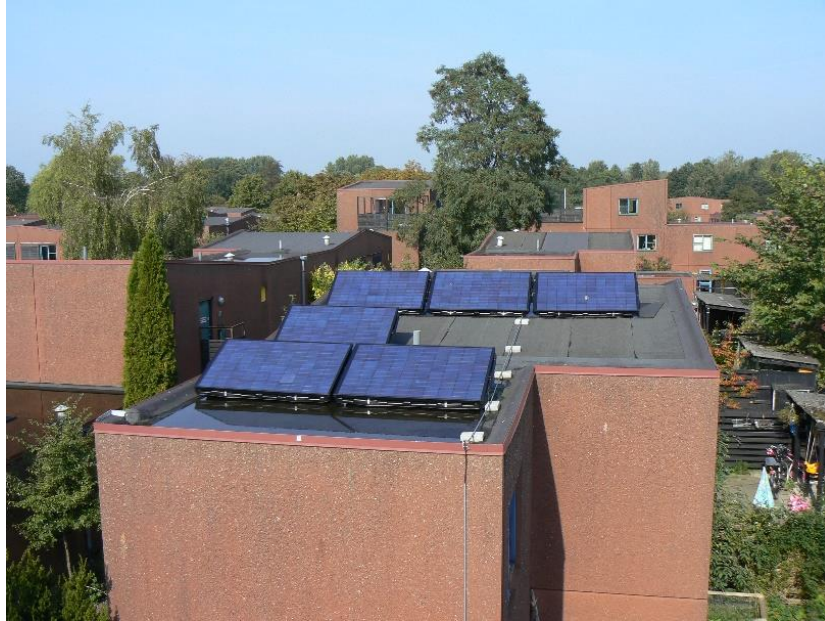
Fig. 25 Additional photovoltaic cells
