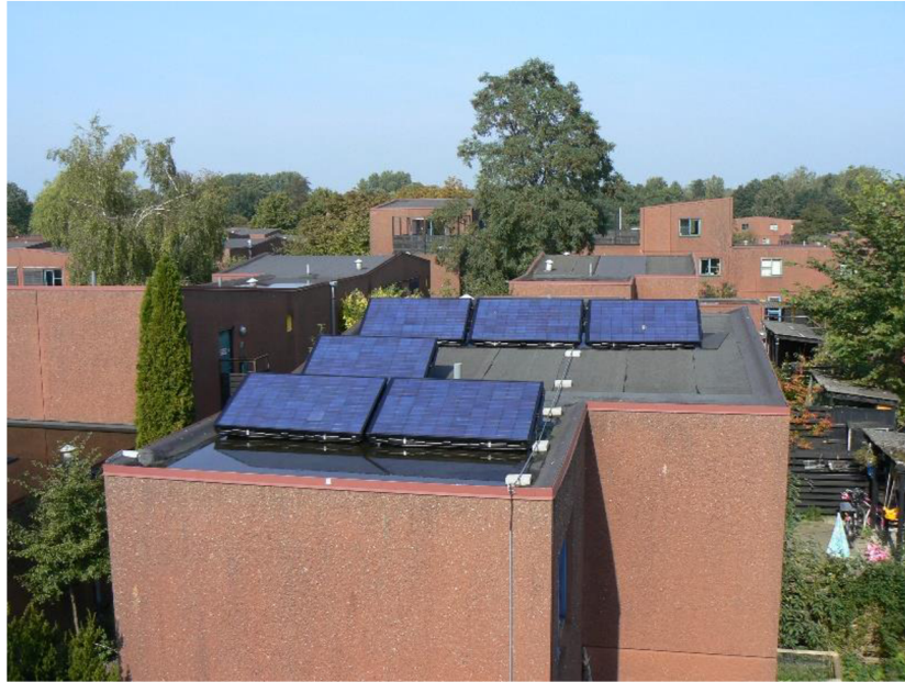
Fig. 25 Additional photovoltaic cells
