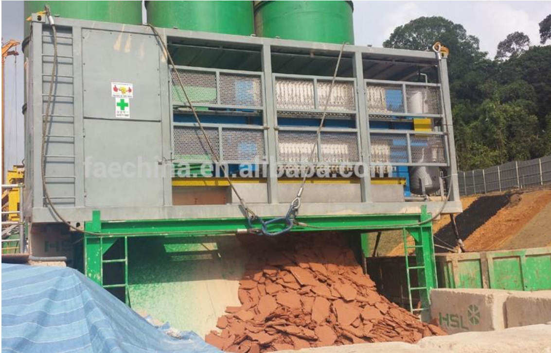
FIGURE 6: EXAMPLE OF THE PLATE AND FRAME PRESS SYSTEM IN USE.
