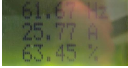
Fig. 5.9 Current data from the frequency converter on frequency, current and the percentage of nominal torque used by the drive system
