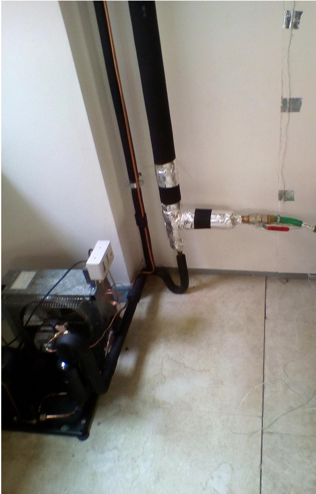
Figure 8.2D – Photo of compressor section (left down) and bottom outflow of refrigerant from evaporator tube at 6 th April 2017.
