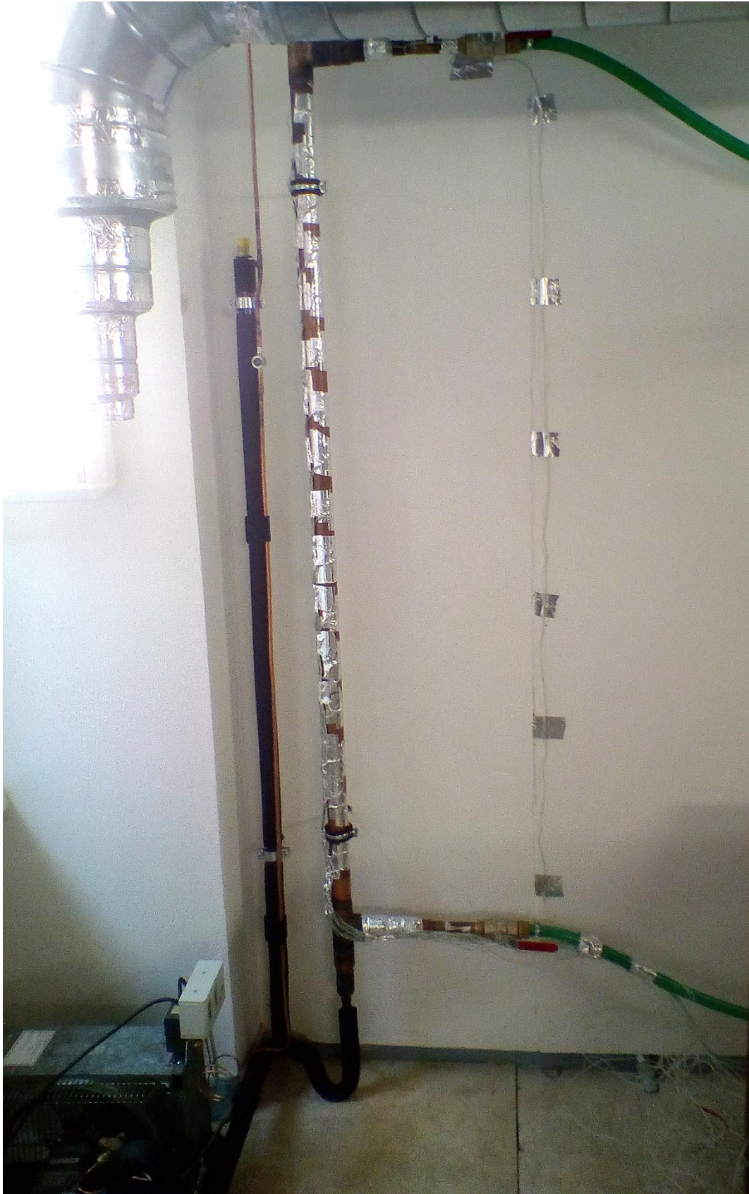
Figure 8.2B – Photo of evaporator tube at 6 th April 2017.
