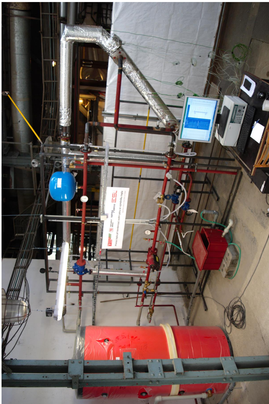
Figure 8.1D – Photo of vertical heat exchanger in parallel-flow at 20 th June 2017.
