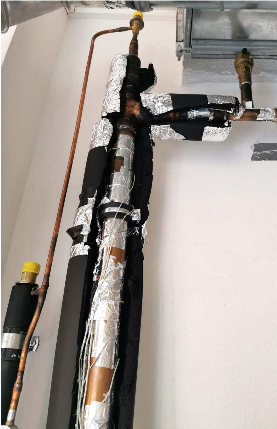
Figure 8.2C – Photo of expansion valve to evaporator tube and upper connection of heating water at 6 th April 2017.
