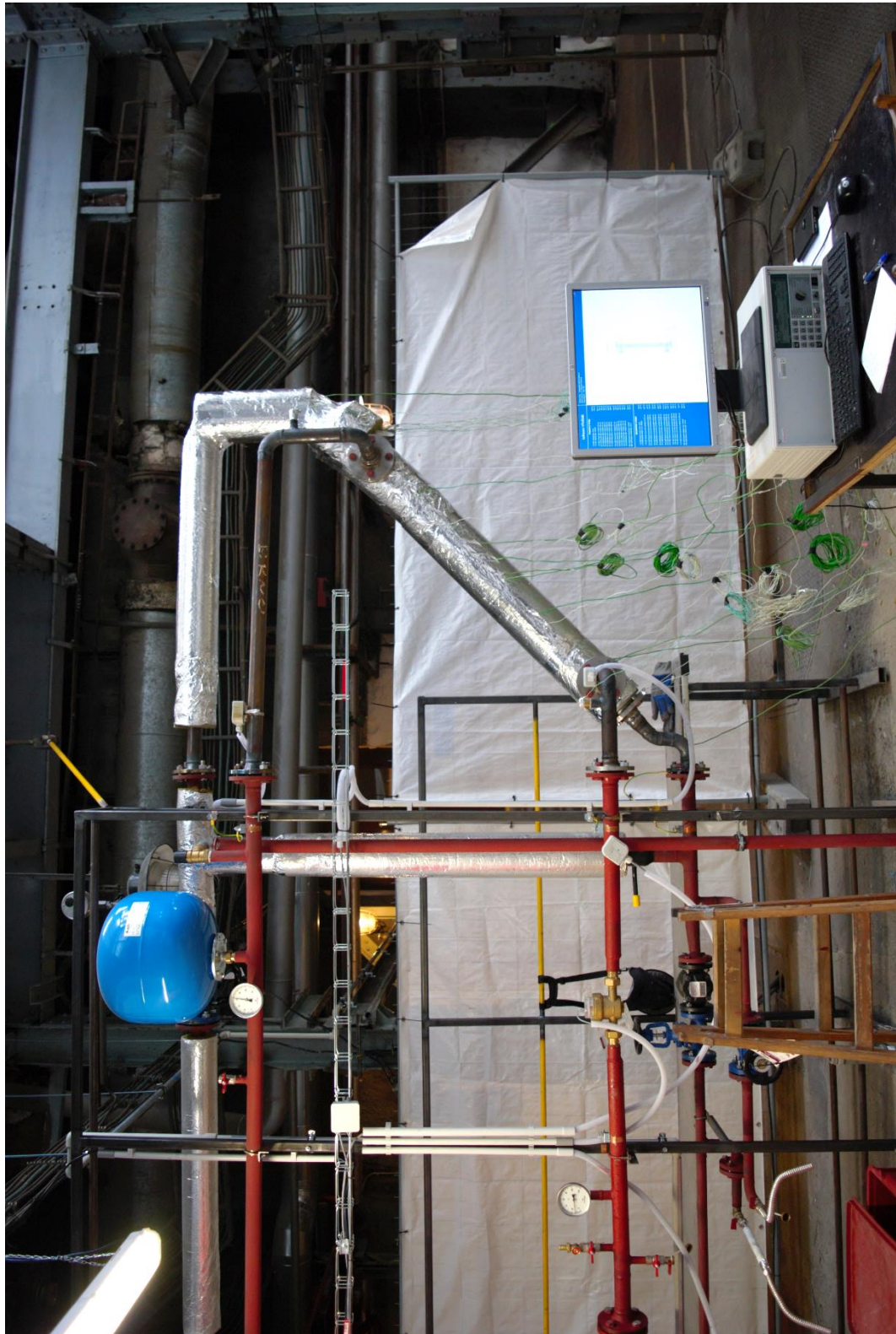
Figure 8.1C – Photo of inclined heat exchanger in counter-flow at 30 th April 2017.
