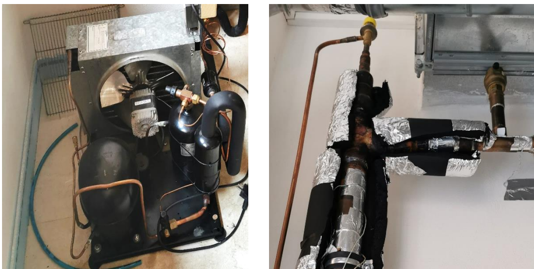
Figure 5.3 – Compressor unit (left photo) and expansion valve (right photo).
