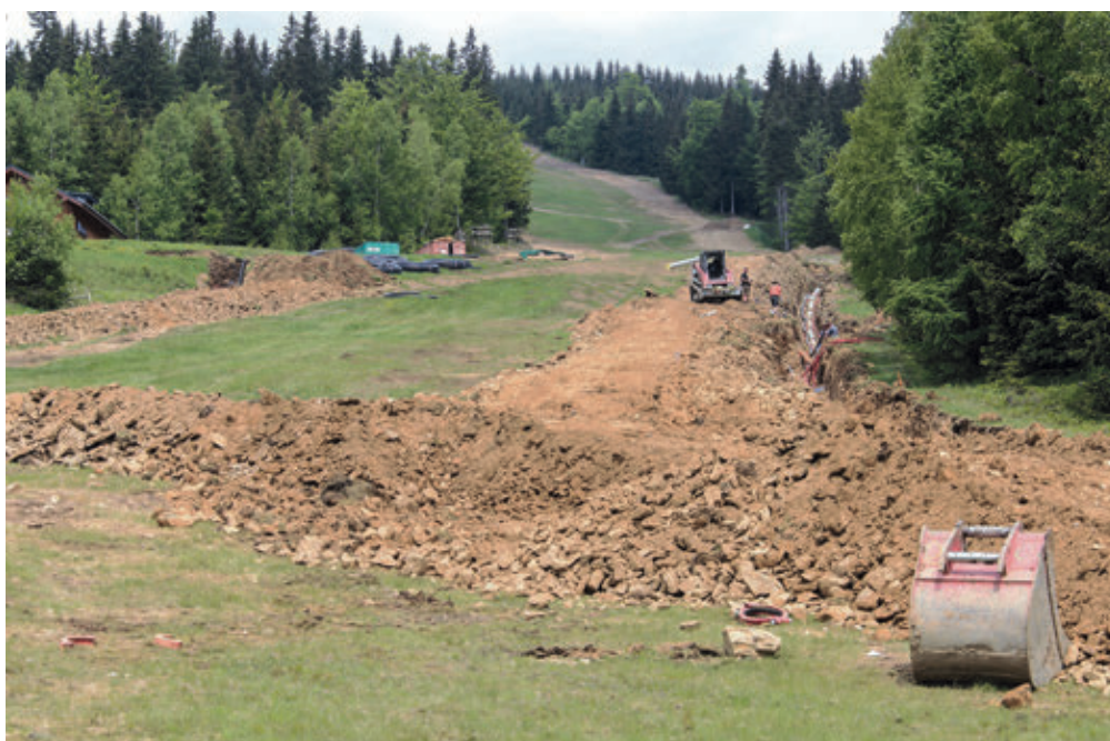
Figure 11. Water pipeline system excavation for water distribution for snowmaking in Medvědin, Špindlerův Mlýn Source: Petr Flousek (27. 5. 2016)
