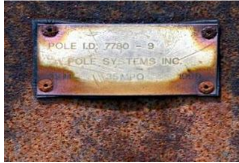
Figure 1.18: Galvanic corrosion of stainless steel plate connected with carbon steel structure. [40]
