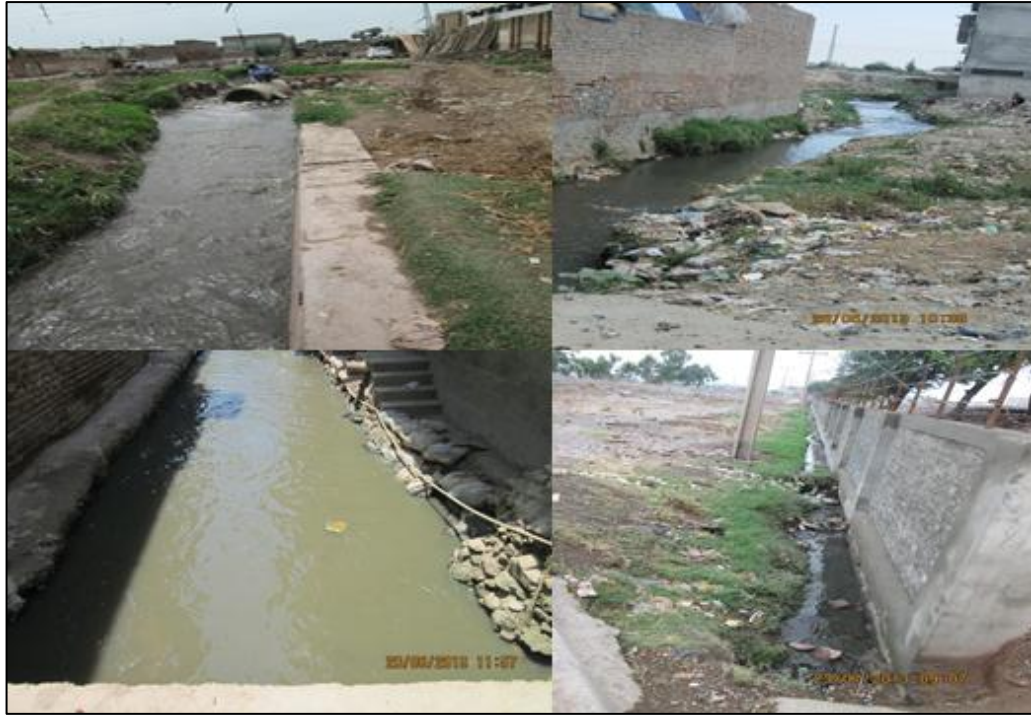
Figure 7: Condition of Stormwater drainage network system.
