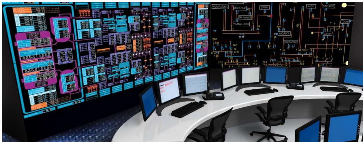
Figure 8 SCADA control system (CTI Supply, 2020)
