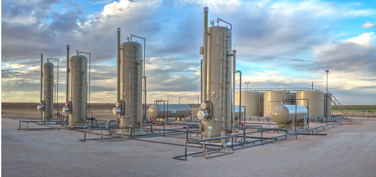
Figure 2 2-Phase Separator (Mashood, 2020)
