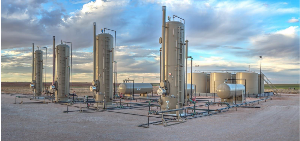
Figure 2 2-Phase Separator (Mashood, 2020)
