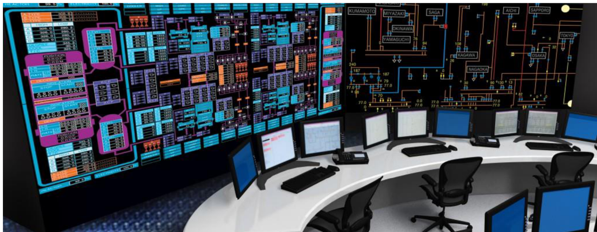
Figure 8 SCADA control system (CTI Supply, 2020)
