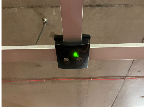
Fig. 1.2: Ultrasonic sensor in a parking garage mounted on a ceiling
