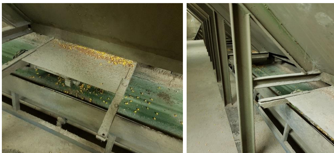
Fig. 5.1: Belt Conveyor measuring point under the income bin (Photo by author, 2023)
