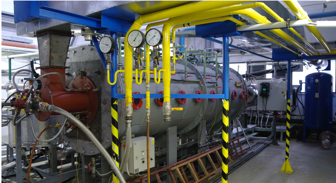
Figure 3-2 Combustion test facility
