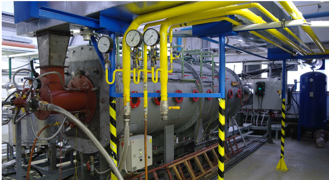
Figure 3-2 Combustion test facility
