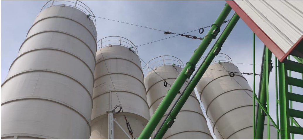
Figure 4: Cement Silo in The Organisation [20]
