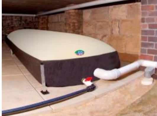
Fig. 12 Bladder water storage tank (45)
