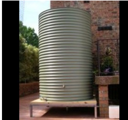
Fig. 10 Steel water storage tank (43)
