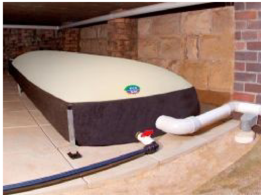
Fig. 12 Bladder water storage tank (45)
