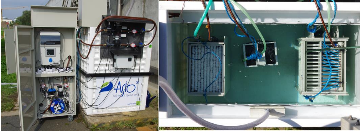
Figure 66: Photo on the left is a cabine with switchboard and PLC control unit with a record. The left image shows the membrane modules during the relaxation phase before starting the test. (Photo, M. Došek)
