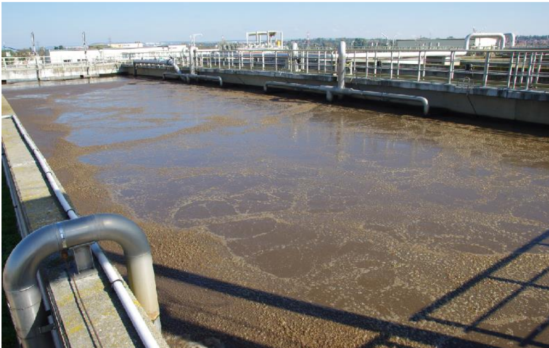
Figure 60: View to the tank with activated sludge, from which was pumped the sludge to a smaller experimental tank. (photo: author)
