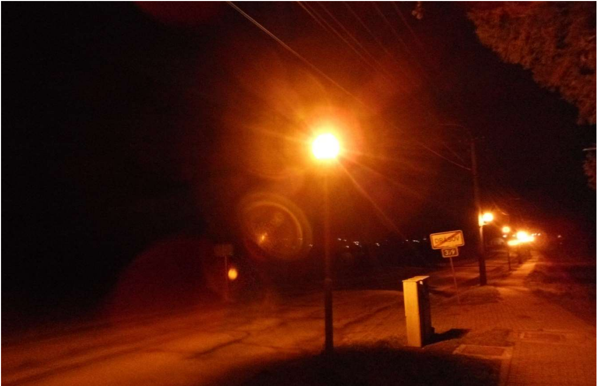
Figure 4. Poorly designed street light that can dazzle drivers.
