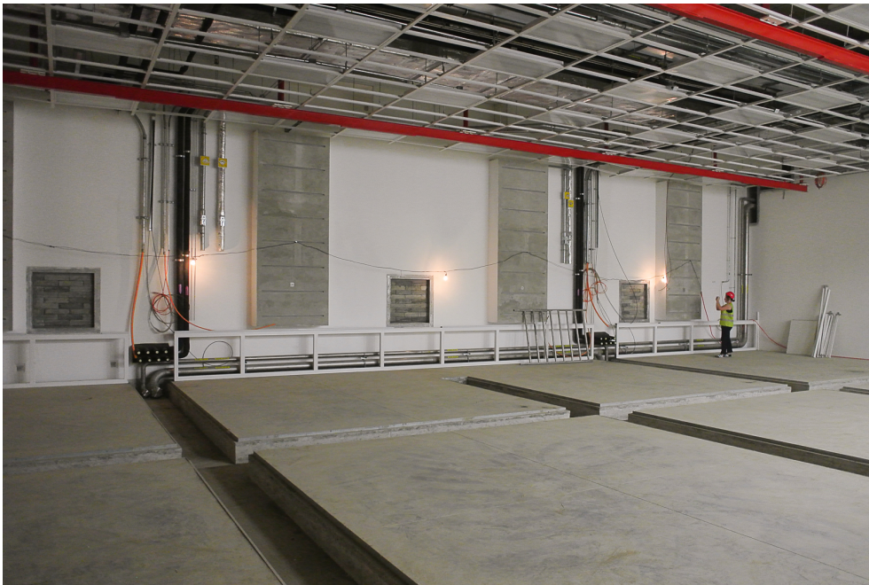
Photo 4: Inside the forthcoming laser hall.
