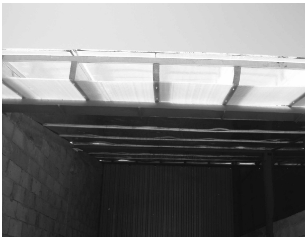
Fig. 5. Detail of solar roof
