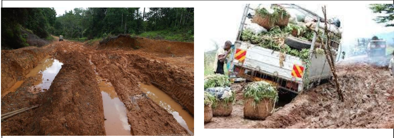
Figure: 22. The bad nature of some forest roads in Ghana
