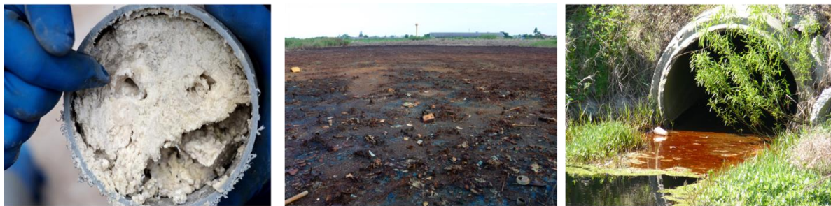
Blockages in pipes
