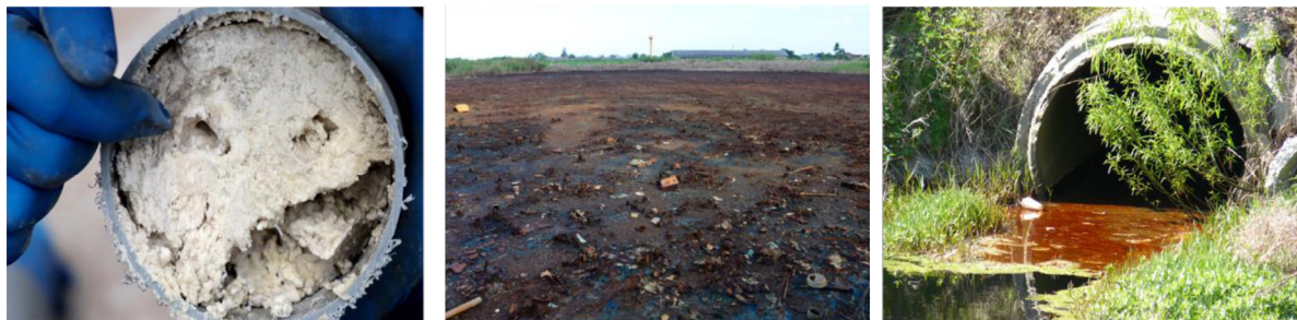
Blockages in pipes
