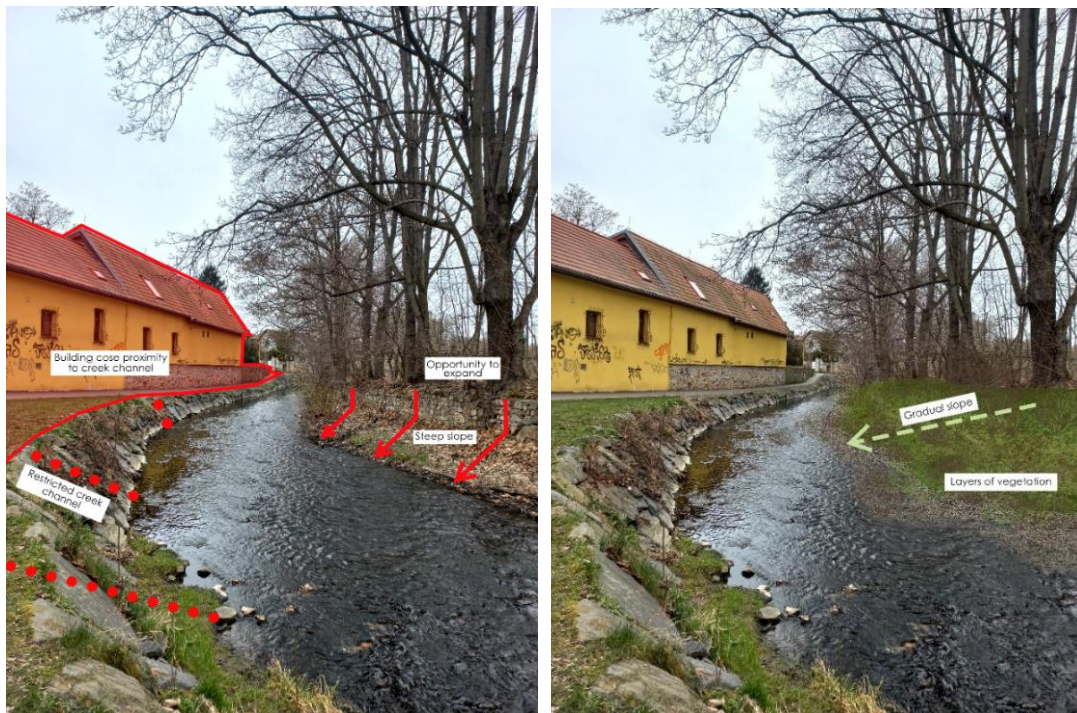
Figure 44. Example 1 – Observed problems at creek channel & Proposed solution close to Hostivařské náměstí. Source: Author
