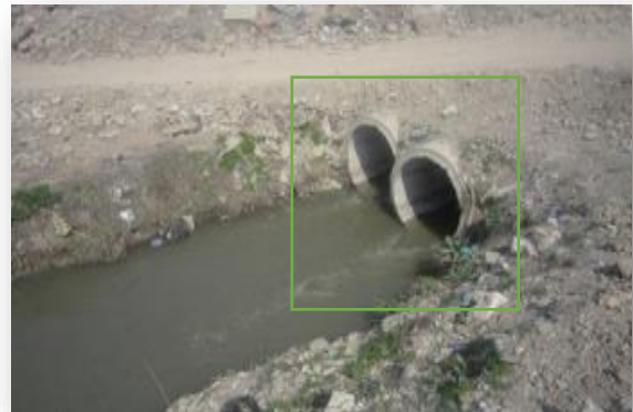
Photo 6.1.4. The pipeline estuary
