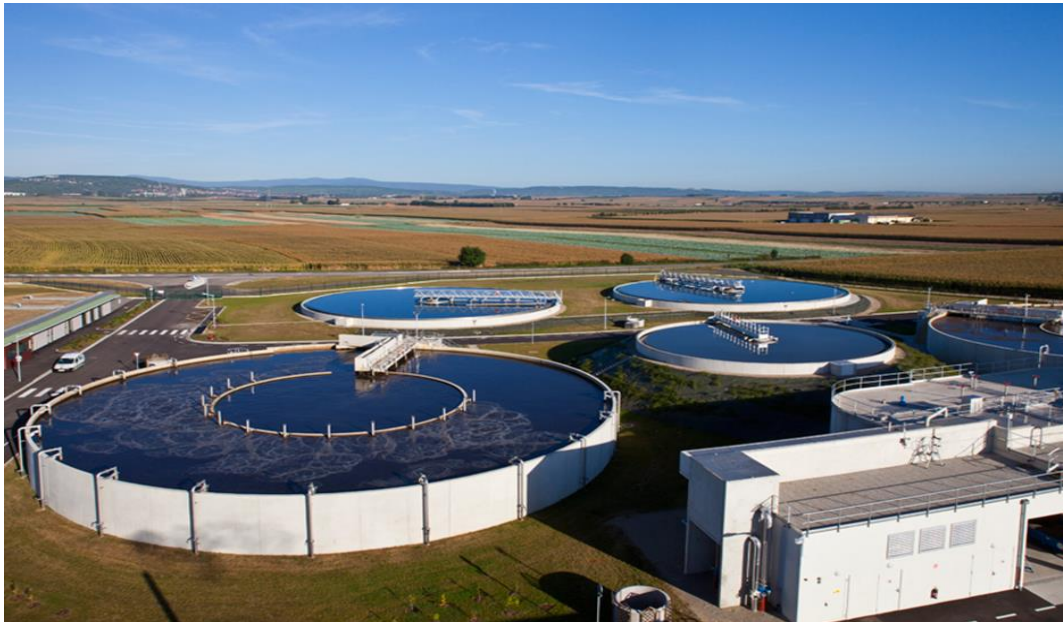
Photo 6.2 of Waste Water Treatment of Meistraizheim
