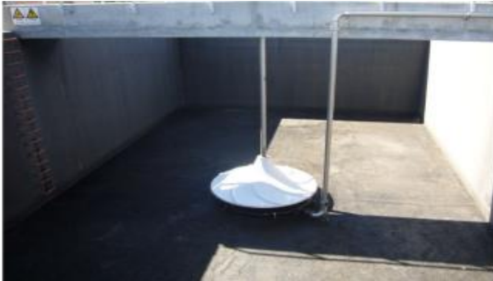
Photo 5.5. Tank Reactor Design
