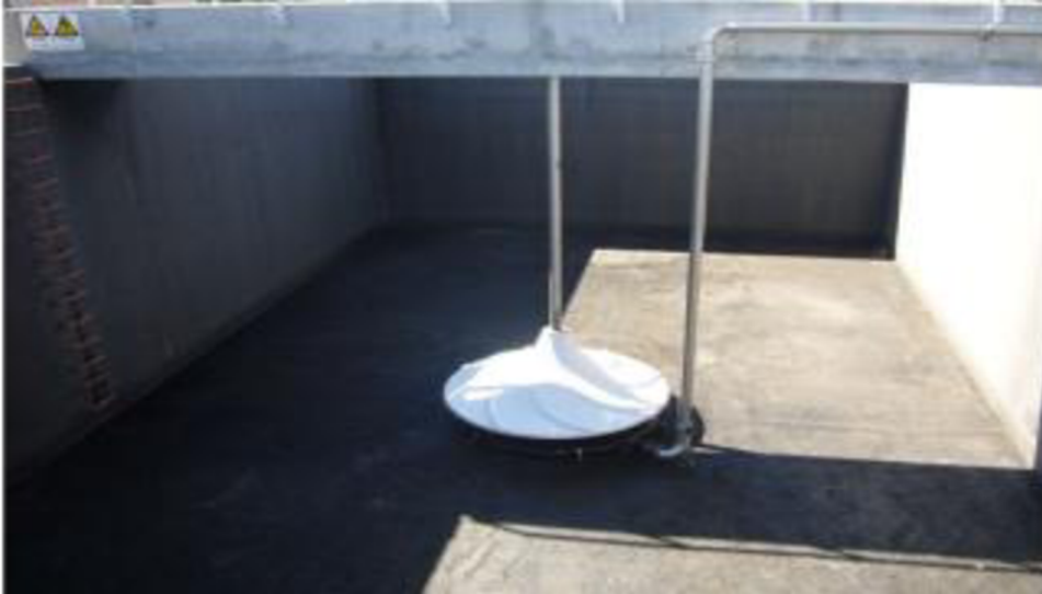
Photo 5.5. Tank Reactor Design
