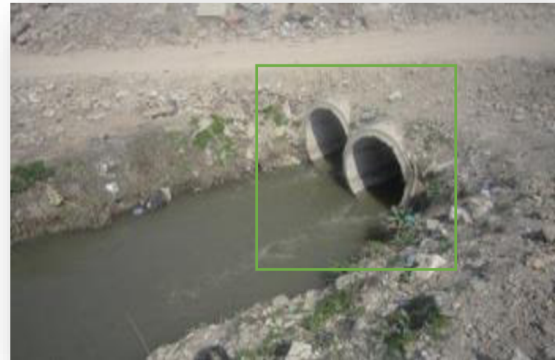
Photo 6.1.4. The pipeline estuary
