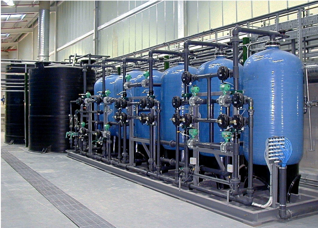
Figure 13 DI Water Recycle Ion Exchange System
