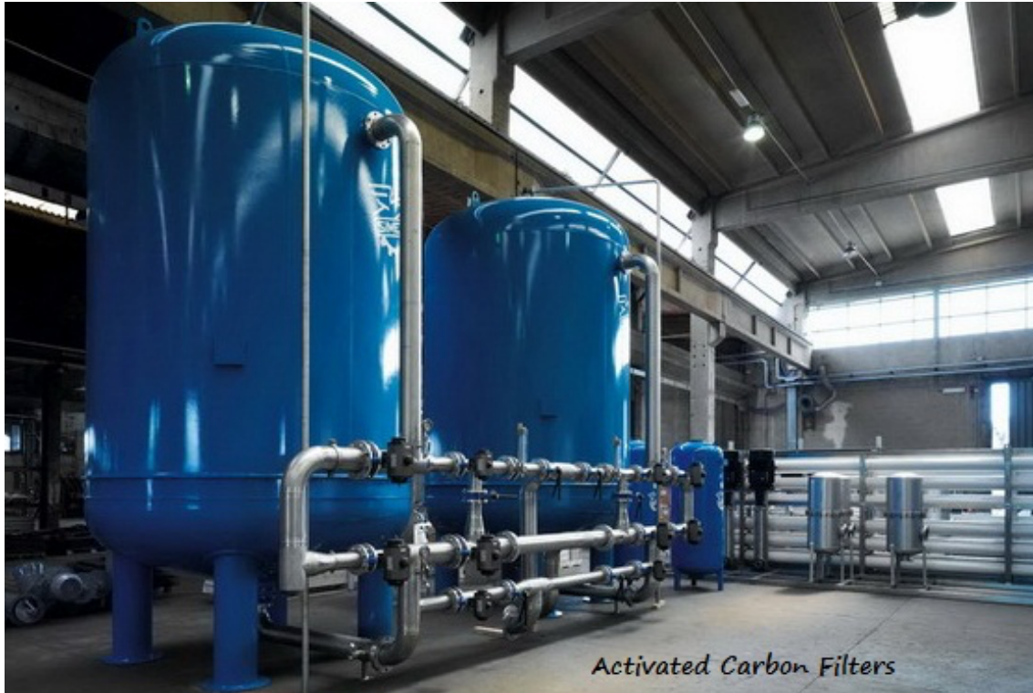
Figure 18 Activated Carbon Filters
