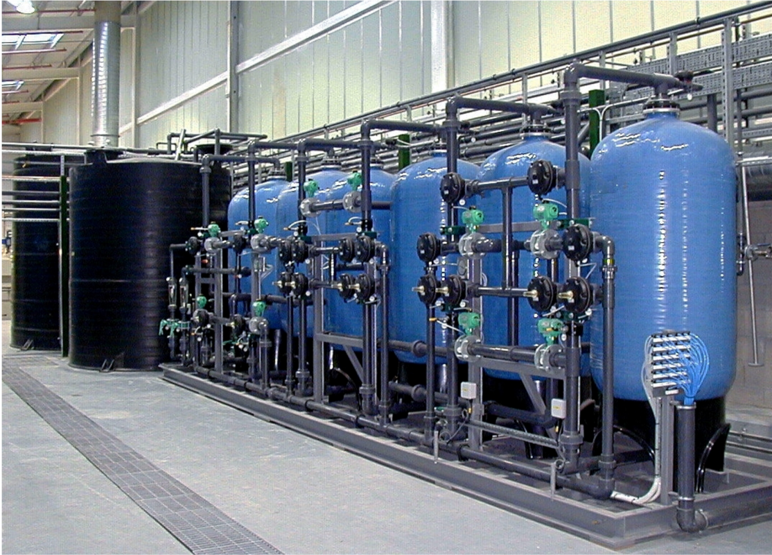
Figure 13 DI Water Recycle Ion Exchange System
