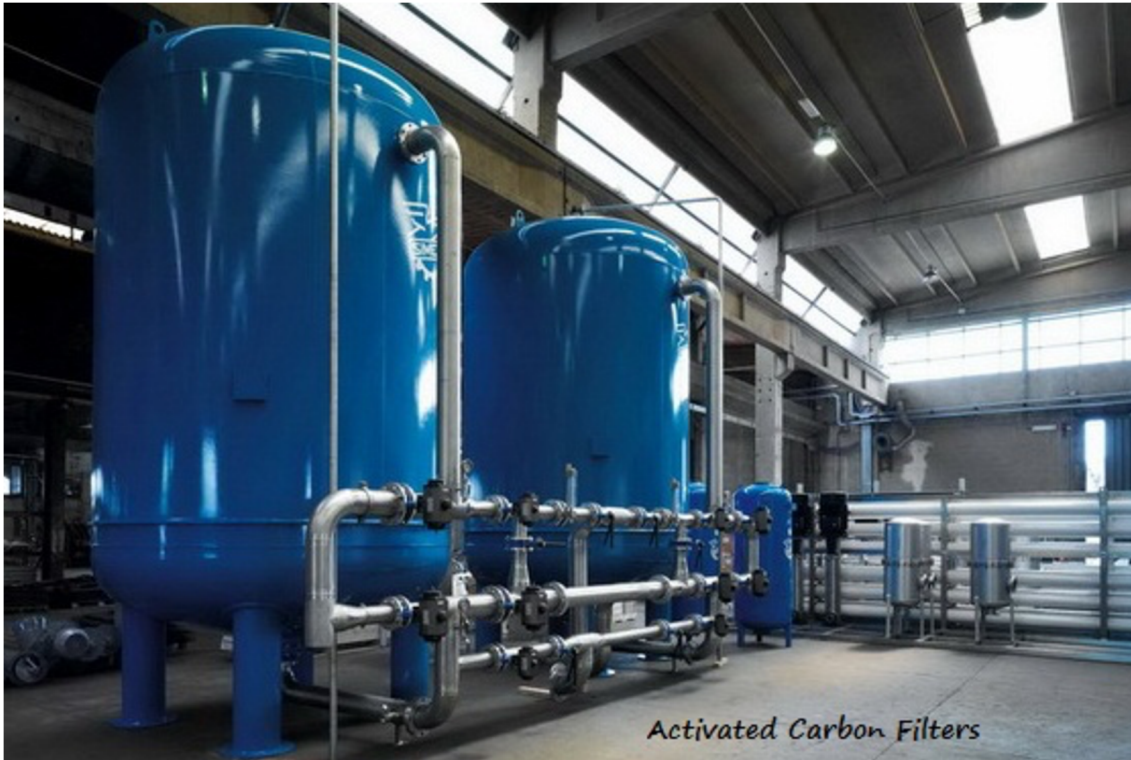
Figure 18 Activated Carbon Filters
