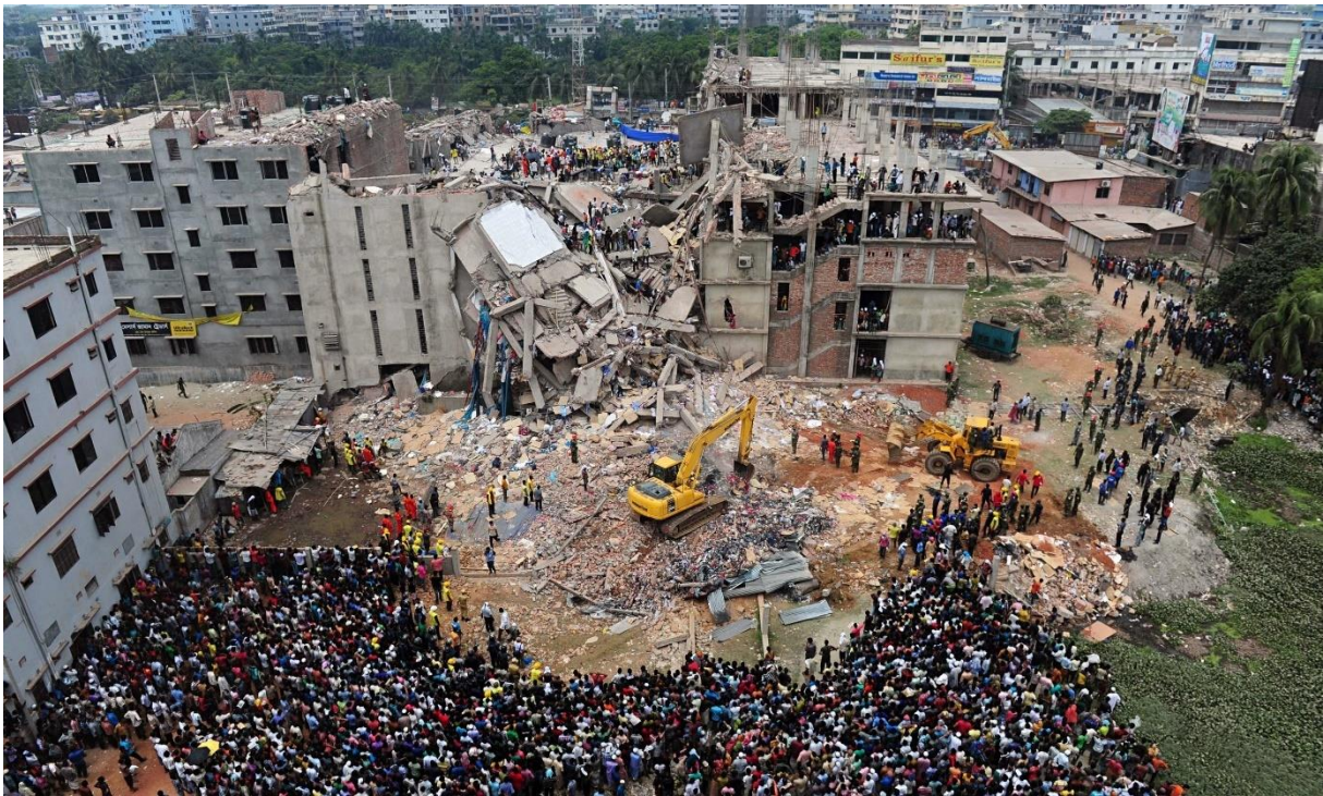
Figure 4: Aerial view of the Rana Plaza building site after it collapsed in April 2013
