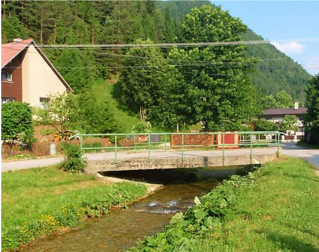
Picture 7. A typical concrete river-bank fortification around a bridge in the E02 section
