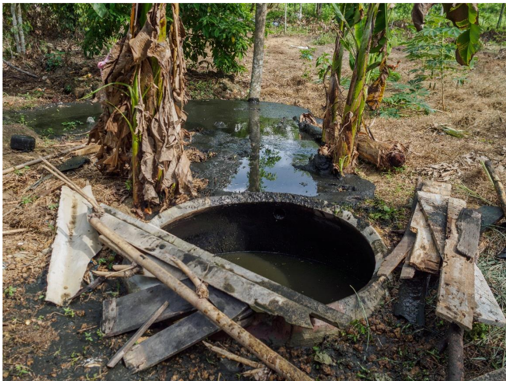
Figure 3 Digestate floating out of the outlet.
