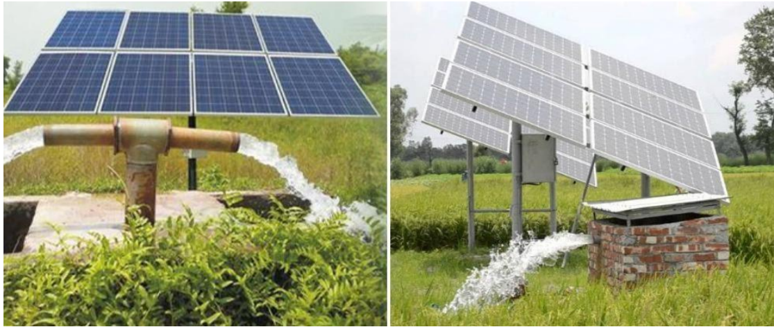
Figure 3: Solar Drip Irrigation System.
