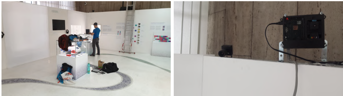
Figure 7.2: Illustration of the thermal unit installation process in the Czech National Museum in Prague.
